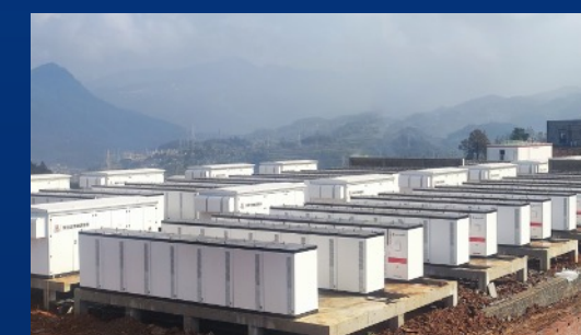
Zhendong Electrochemical 100MW | 200 MWh Energy Storage Project
