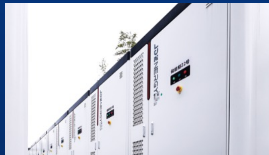
Zhejiang Jinsheng Holding Group Co., Ltd. 11MW/22MWh Energy Storage Power Station
