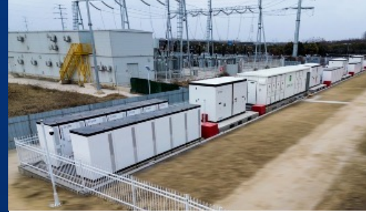
Tongwei Yancheng 10MW/20MWh Energy Storage Station
