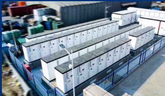
Hefei TCL Home Appliances 10MW/20MWh Energy Storage Station
