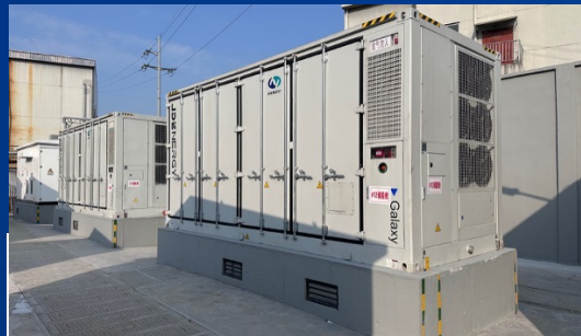
Hengyi Petrochemical 33.5 MW | 67 MWh Energy Storage Project
