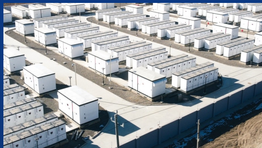
Niushoushan 200MW/400MWh Energy Storage Power Station Project
