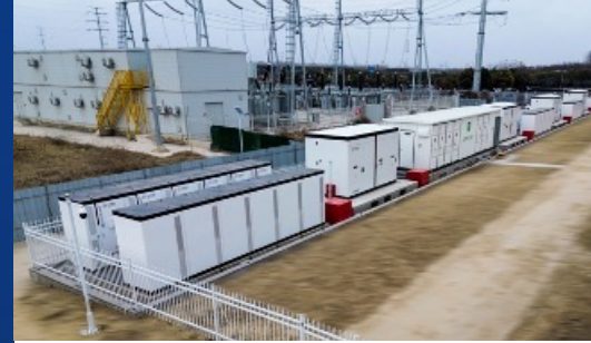
Tongwei Yancheng 10MW/20MWh Energy Storage Station
