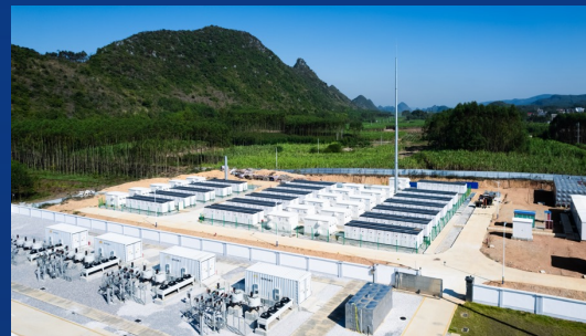
Guangxi Guigang 144MW/ 288MWh Energy Storage Station Project
