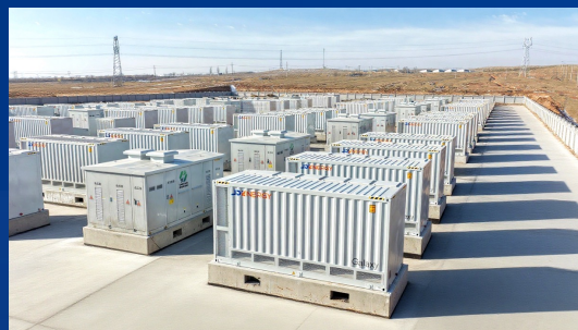
Ningxia Hanjun 150 MW | 600 MWh Energy Storage Project
