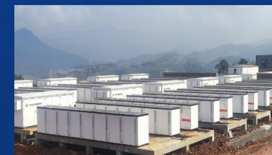
Zhendong Electrochemical 100MW | 200 MWh Energy Storage Project
