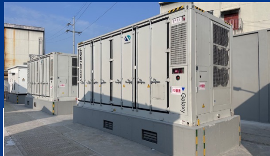
Hengyi Petrochemical 33.5 MW | 67 MWh Energy Storage Project
