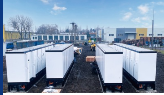
Hungary Industrial and Commercial 6MW/12MWh Energy Storage Project
