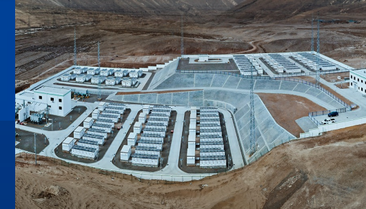
Ningxia Huayan Substation 200MW/400MWh Energy Storage Power Station
