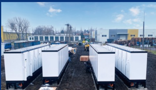
Hungary C&I 6MW/12MWh Energy Storage Project
