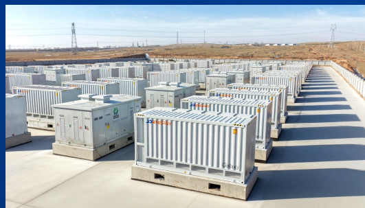
Ningxia Hanjun 150MW/600MWh Energy Storage Project
