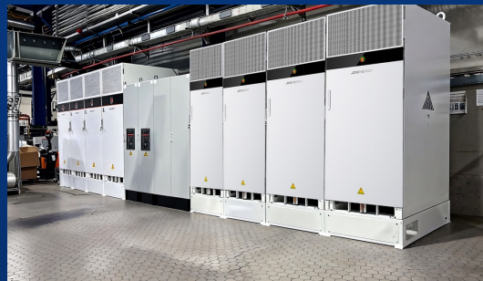
Germany Oldenburg C&I 2MW/4MWh Energy Storage Project
