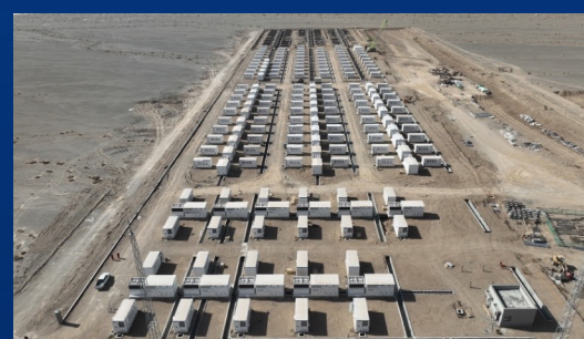
Gansu Jiuquan 450MW/900MWh Energy Storage Project
