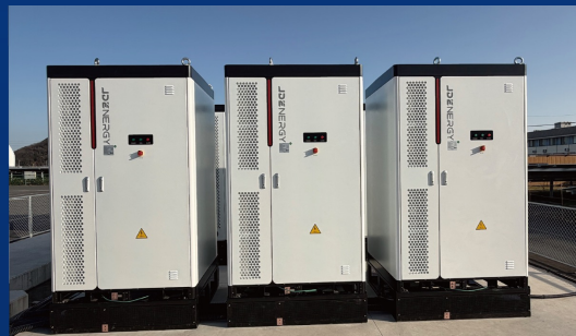
Japan C&I 1.29MW/2.508 MWh Energy Storage Project
