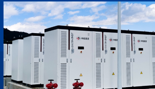
CNNC Lin Xiang 200MW/400MWh Energy Storage Power Station
