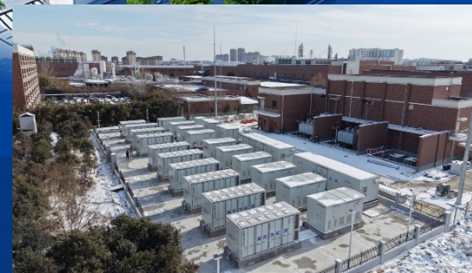
Jiangsu Huai'an Industrial and Commercial 25 MW/50MWh Energy Storage Project
