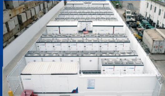
Shenzhen Chiwan port 16MW/60MWh Energy Storage Demonstration Project
