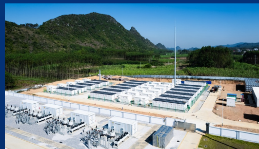
Guangxi Guigang 144MW/288MWh Energy Storage Station Project
