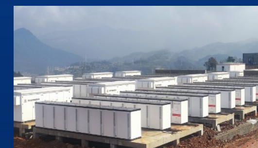
Zhendong Electrochemical 100MW/200 MWh Energy Storage Project
