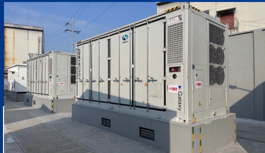
Hengyi Petrochemical 33.5MW/67MWh Energy Storage Project
